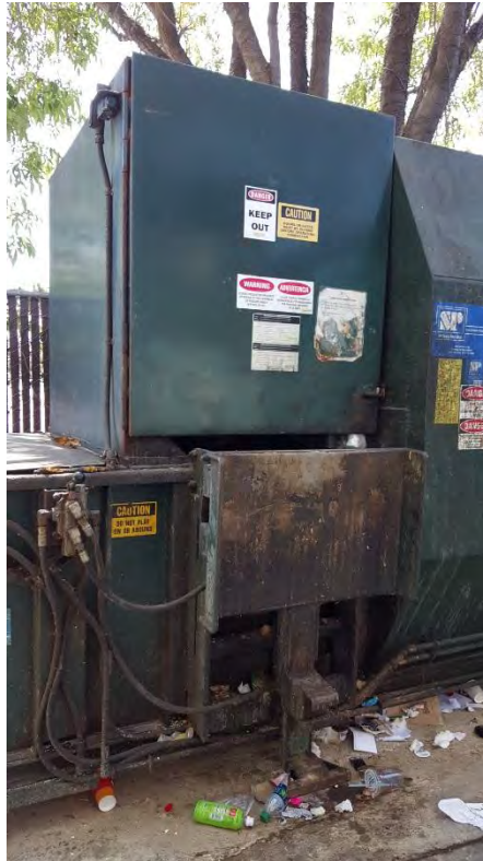
PHOTO #26. TRASH COMPACTOR.
