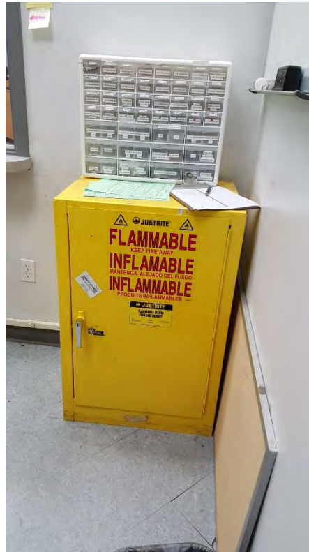
PHOTO #11. CHEMICAL STORAGE AT THE SHANE COMPANY.
