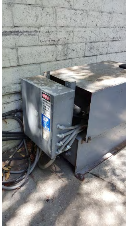
PHOTO #27. POWER FOR TRASH COMPACTOR.
