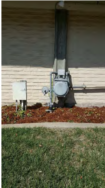
PHOTO #28. ELECTRICAL METER.
