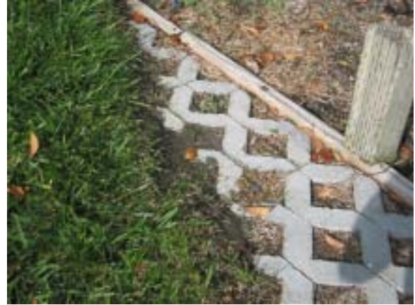
Close-up picture shows the concrete turf block matrix not covered in grass.
